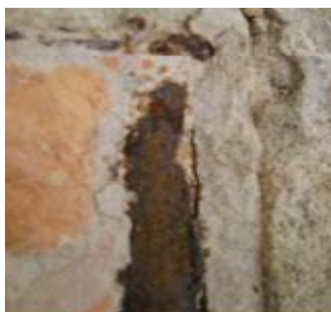
Figure 5. Columns' longitudinal reinforcement eroded (corrosion).
