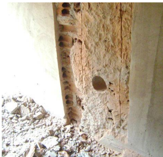
Figure 4. Testimonies' extraction hole in a column.
