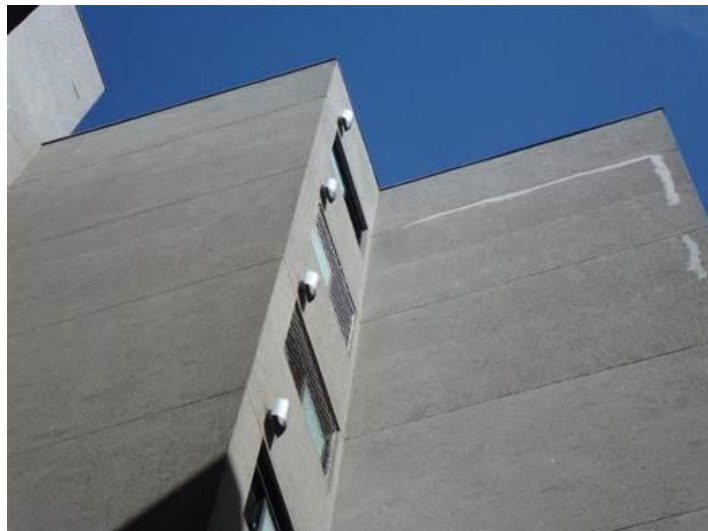
a) Thermal variation fissures.
