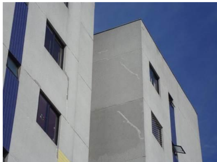
b) Structure movement fissures.
