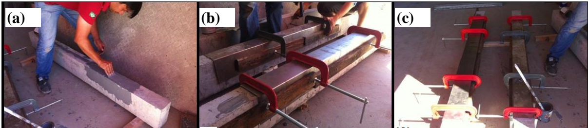
Figure 4. (a) Application of the epoxy adhesive to anchor the steel profiles; (b) Placement of the fasteners; (c) Final fastening system of the sheets.
