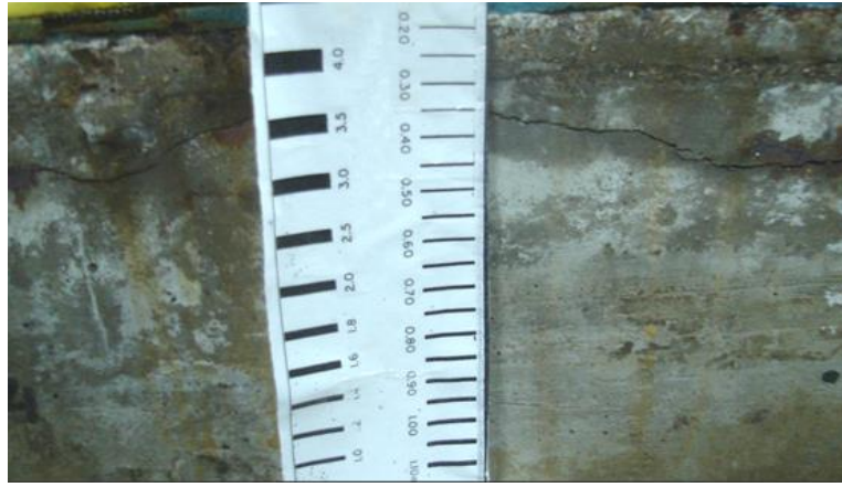
Figure 2. Measurement of the width of a crack generated by accelerated corrosion.
