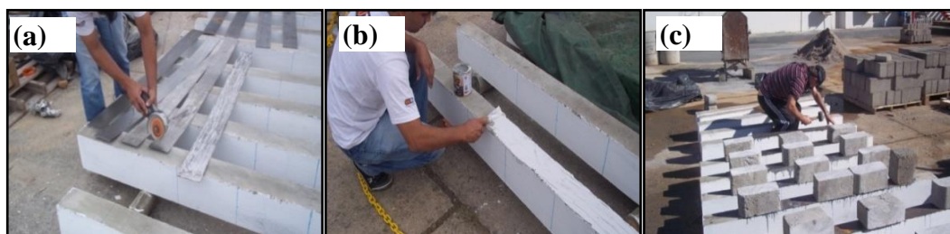
Figure 3. (a) Preparation of the sheets; (b) Application of the epoxy structural adhesive; (c) Fixing and support of the sheets.
