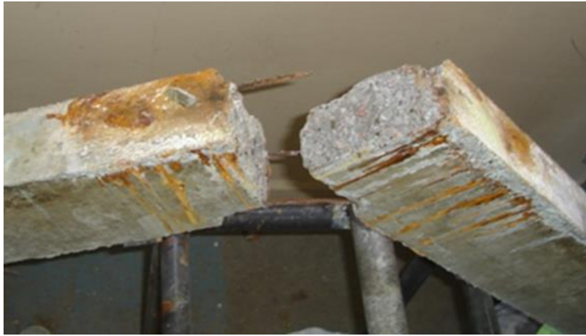
Figure 4. Beam V96 after collapse
