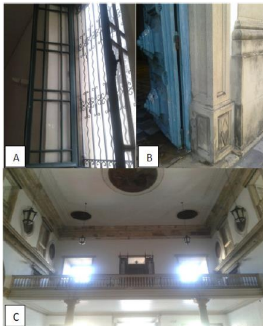
Figure 3. Absence of vertical compartmentalization within the Madre de Deus´ Church. A – Balcony and windows inside the church; B – Ladder of the common type; C – Balcony inside the building itself.
