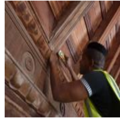
Figure 23. Measurement of superficial humidity on elements.
