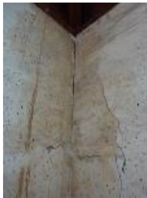
Figure 14. Crack 1-2 cm thick at the intersection of axes A-1.
