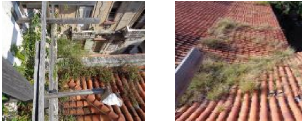
Figure 26 and Figure 27. Invading plants on roof of the High Choir.
