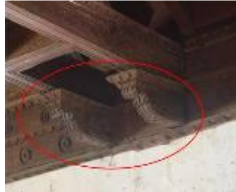
Figure 17. Dropping of corbels under tie rod beams 1 and 2 (T1 and T2), on axis 1.
