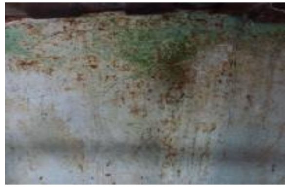
Figure 10. Top wall green patinas in axis 2.
