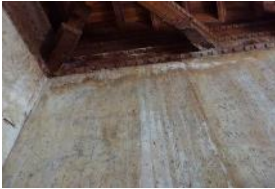
Figure 9. Wall with rain wash in axis A
