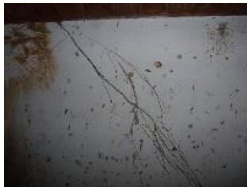
Figure 11. Roots in axis A from the feeder plants on the roof.
