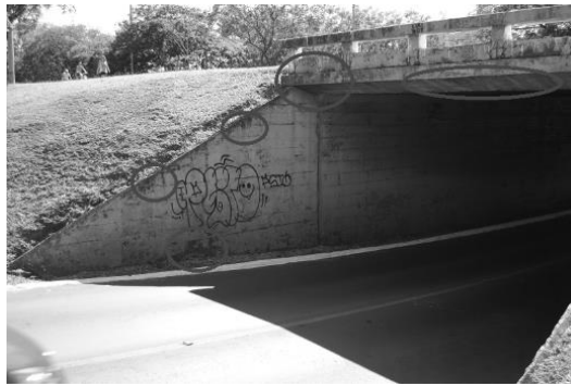
Figure 6. Stains scattered on the structure
