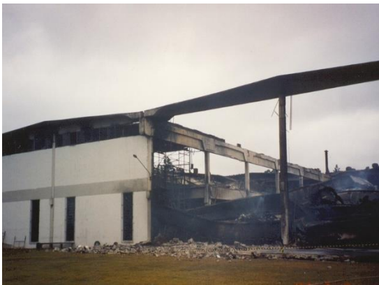
Figure 11. Collapse of building with precast structure subjected to fire
