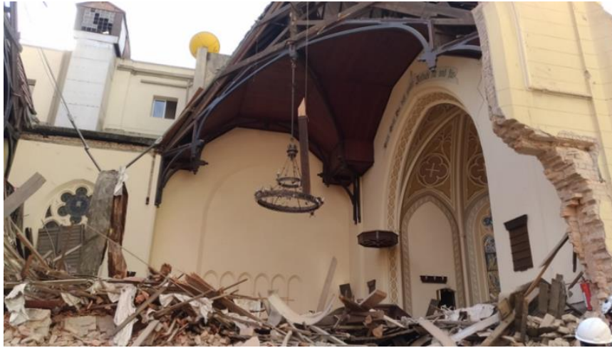
Figure 3. Damage to the Lutheran Church, next to Ed. Wilton Paes de Almeida (source: Paulo Helene's personal collection)
