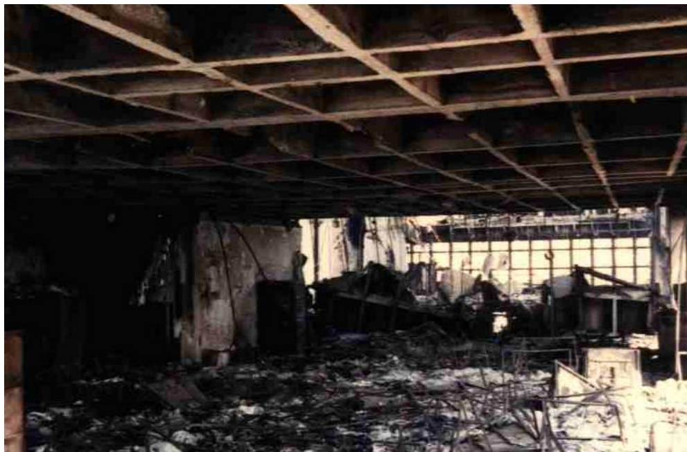
Figure 15. Front view of the Sede II building structure, from its rear, highlighting the void left by the collapse of the central part
