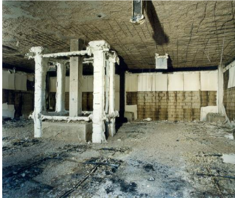
Figure 18. Detail of extent and severity of slab spalling ( f_{ck} = 74 MPa) after fire simulation. Highlighting, observe the integrity conditions of the high strength concrete column ( f_{ck} = 103 MPa) (Chana & Price, 2003).
