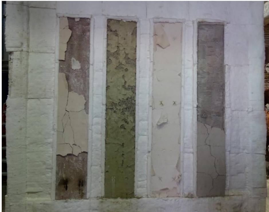
Figure 4. Detail of the elements and coatings condition after furnace opening (event 1): smooth formulated plaster coating, reference element, projected plaster coating and cement-based mortar coating.
