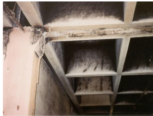
Figure 12. Support displacement of pre-molded fire structure
