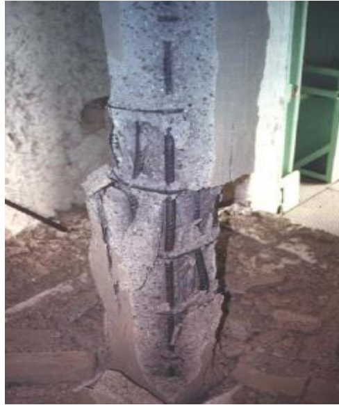
Figure 10. Example of explosive spalling occurred in high strength concrete column f_{ck} = 83 MPa (Kodur et al., 2005).
