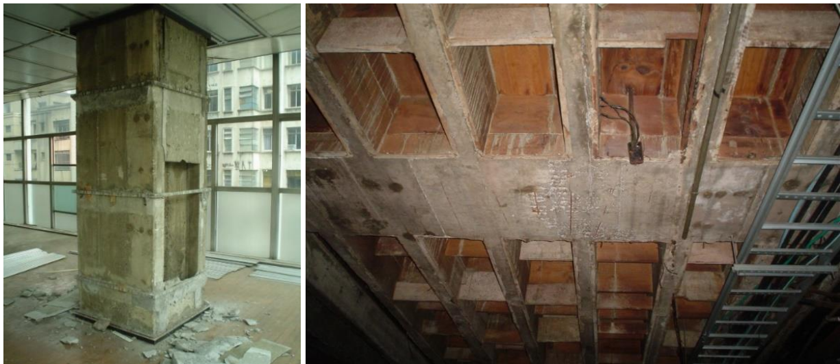
Figure 6. Columns without metal coating, where it is observed the "H" which is actually a shaft of the air conditioner and I grate beam track with AJE still forms wood. (source: personal collection of Leandro Coelho)
