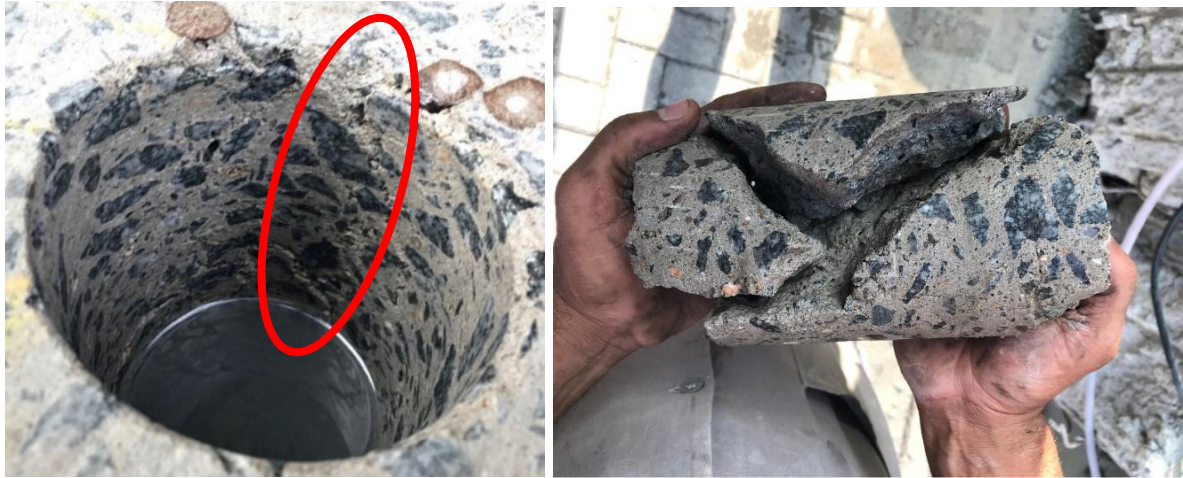
Figure 13. Visible cracks during extraction and decomposed core. (Source: Paulo Helene's personal collection)
